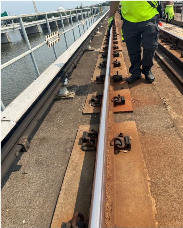
Photo 4: Shows loose washers on fasteners at L2 120+30 to 120+50.
