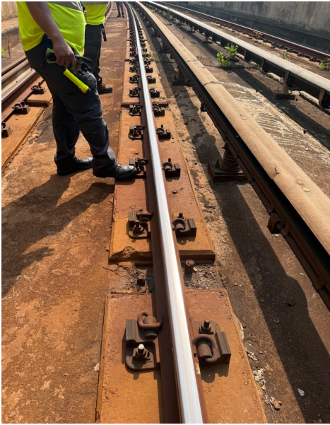
Photo 1: Defective fasteners with loose washers at L2 139+50 to 139+70, left rail.
