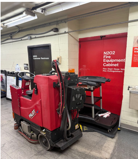
Photo 5: Shows equipment blocking the fire cabinet.
