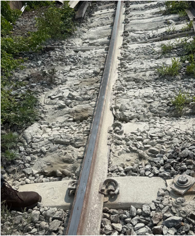
Photo 2: Fouled ballast area at L2 136+50.
