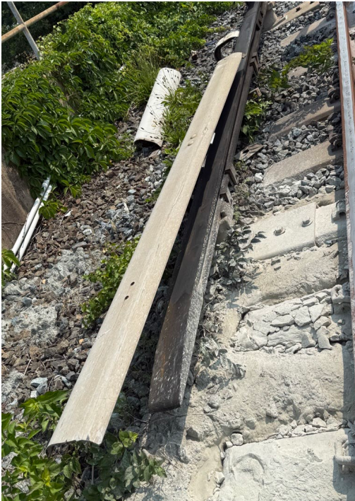
Photo 3: Missing or damaged third rail cover board.
