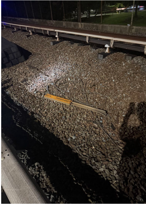
Photo 7: Broken chain marker sign.
