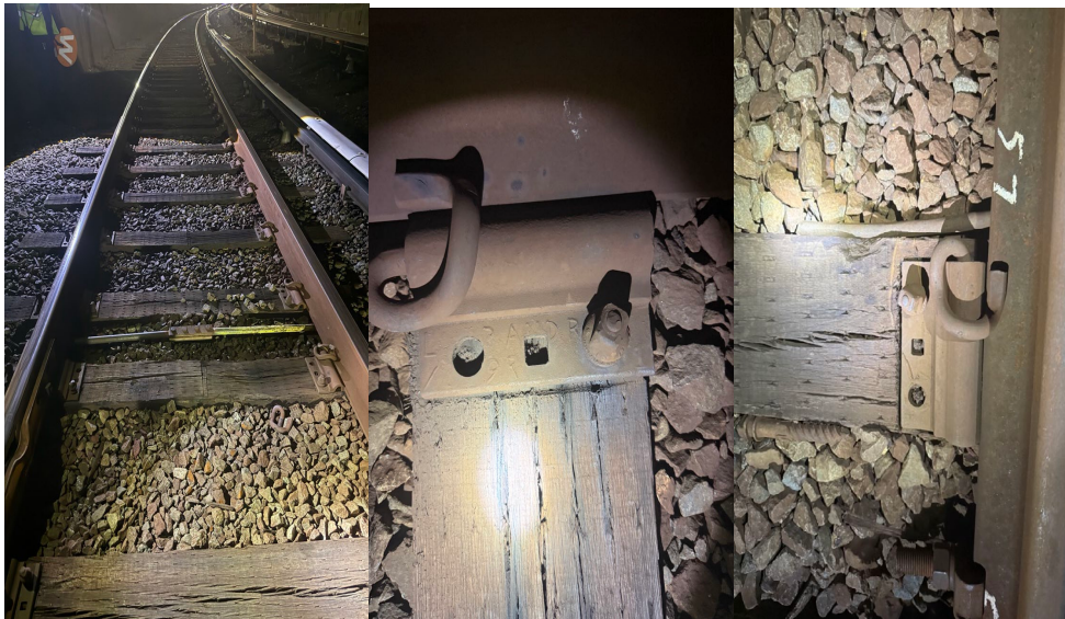
Photo 1 (left): Location of gauge rod at C1 347+50. Photo 2 (middle): Visible lateral movement on the tie plate. Photo 3 (right): Tie plate embedded in the tie, causing tie plate cutting.
