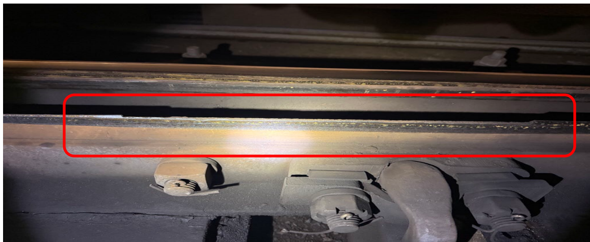
Photo 4: Shows chipping on the switch point on switch 6 at National Airport (C10).
