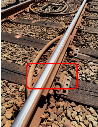
Photo 3: Broken joint bar bolt not secured.
