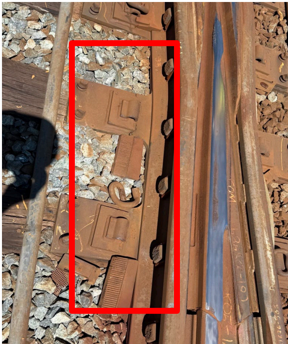
Photo 2: Missing clips on frog plate at 1A switch.
