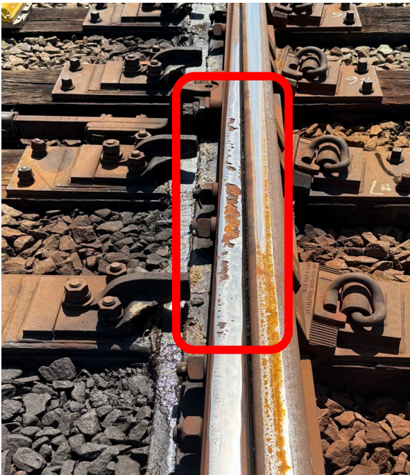
Photo 1: Severe chipping on the switch point at 1b switch.
