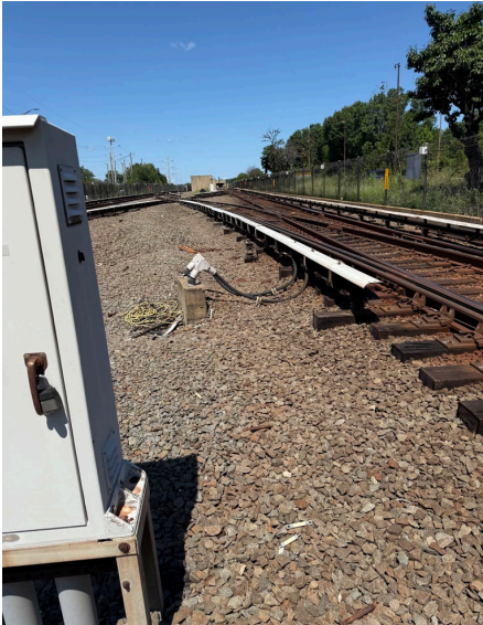
Photo 4: Shows low ballast on the shoulders of the ties.
