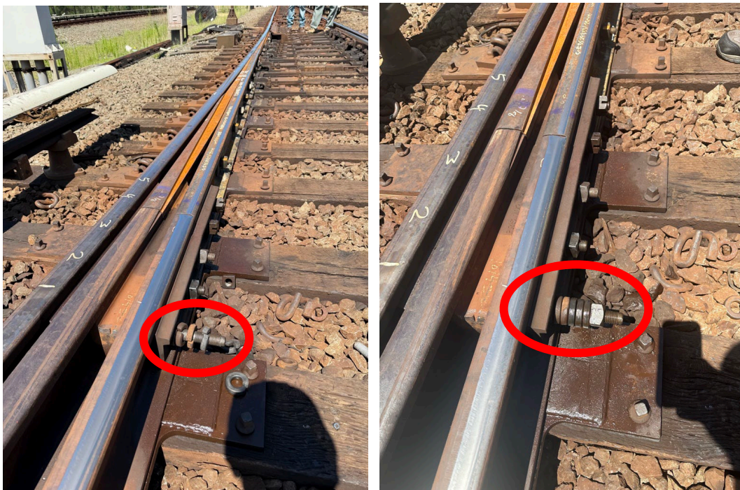
Photo 5 (left): Missing nut and washers on heel block bolt at 3B switch. Photo 6 (right): Shows that temporary repairs were made to secure the bolt.
