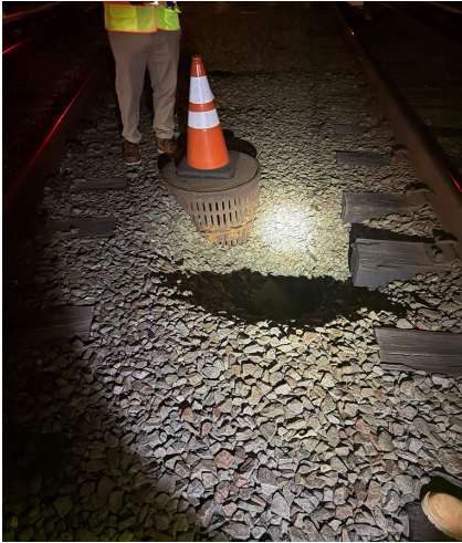
Photo 1: Sinkhole near switch 19 on the outbound end of the pocket track.
