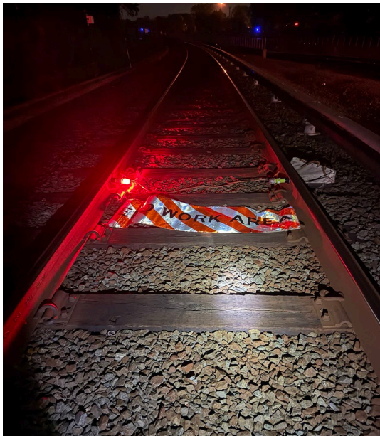
Photo 3: One of the E-flare lights was not illuminated.
