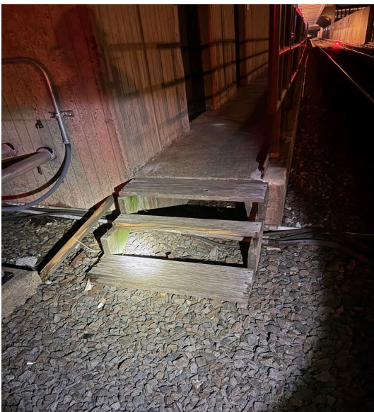
Photo 2: Shows the defective step and the broken board.
