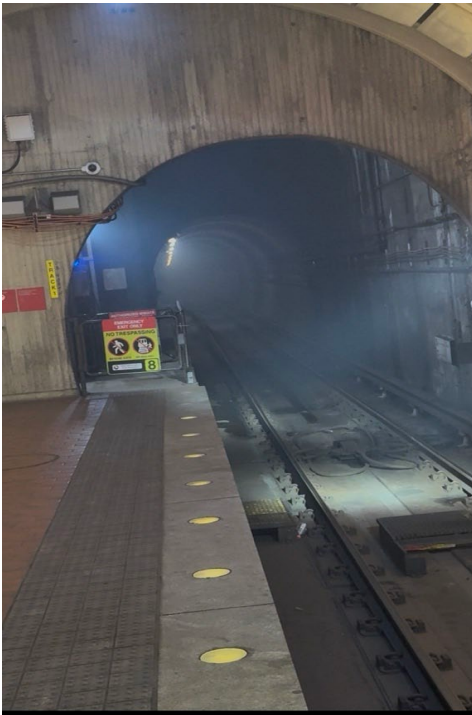
Photo 1: Smoke in the tunnel at Forest Glen (B09) track 2.
