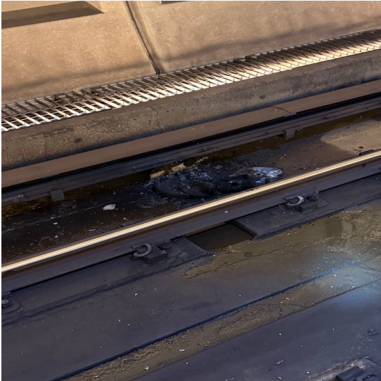
Photo 2: Exploded insulator and grout pad.
