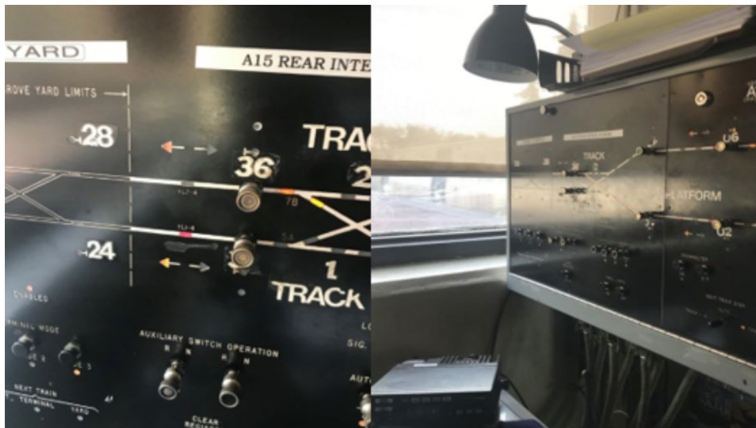
Photo 1 - (left) forward-facing view of control board. (right) - Angle view of control board with sun glare.
