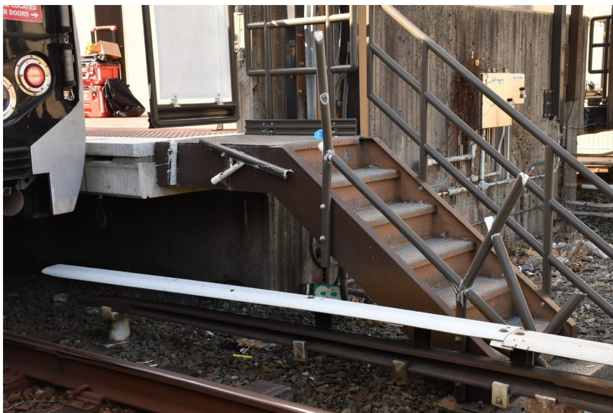
Image 6 - View of the damaged end gate and railing from the track bed.
