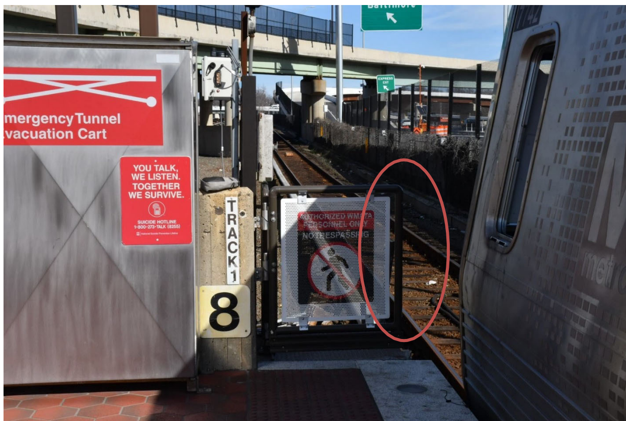
Image 4 - Track 1 end gate. Damaged area circled
