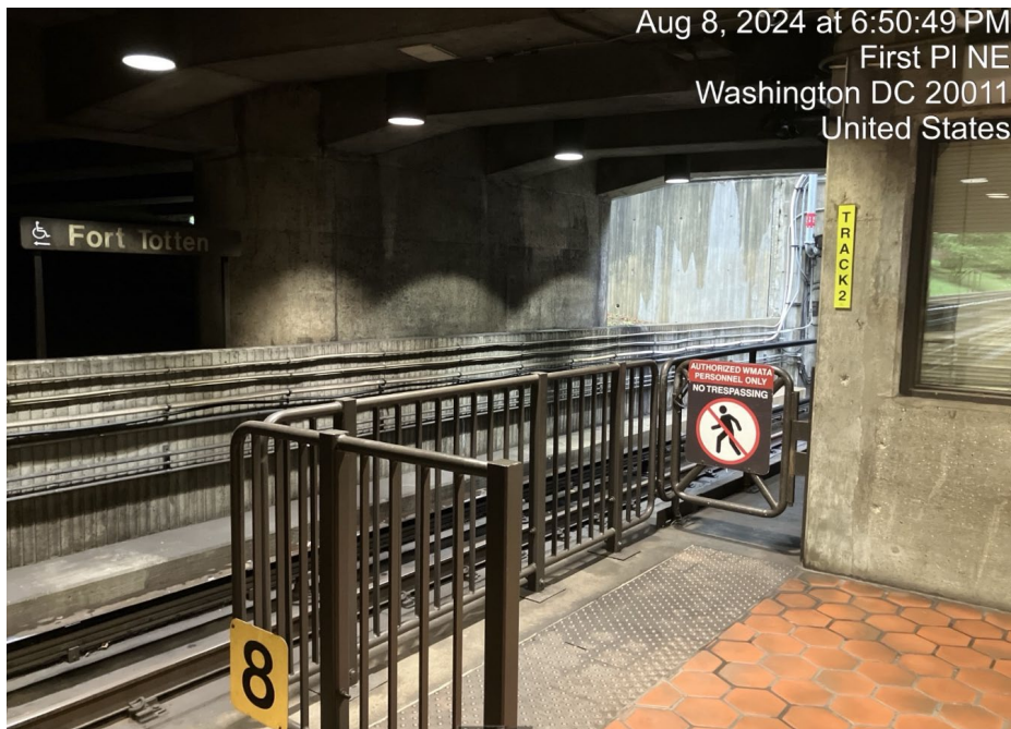
Image 4: End gate of the 8-car marker for track 2 at Fort Totten Station.
