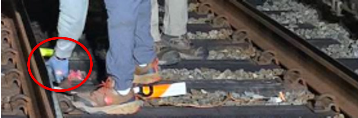
Photo 2: Personnel not wearing Class O rubber insulated gloves (PPE) to install shunts.
