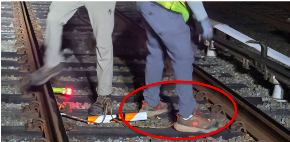
Photo 1: Non-compliant footwear being used while on the roadway performing job duties.
