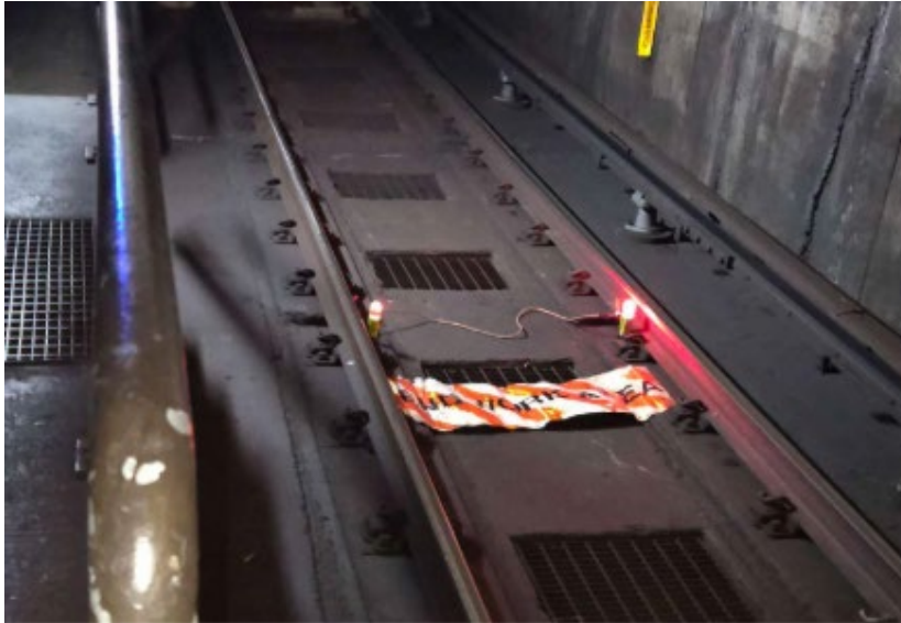
Photo 9: Compliant ETO setup.
